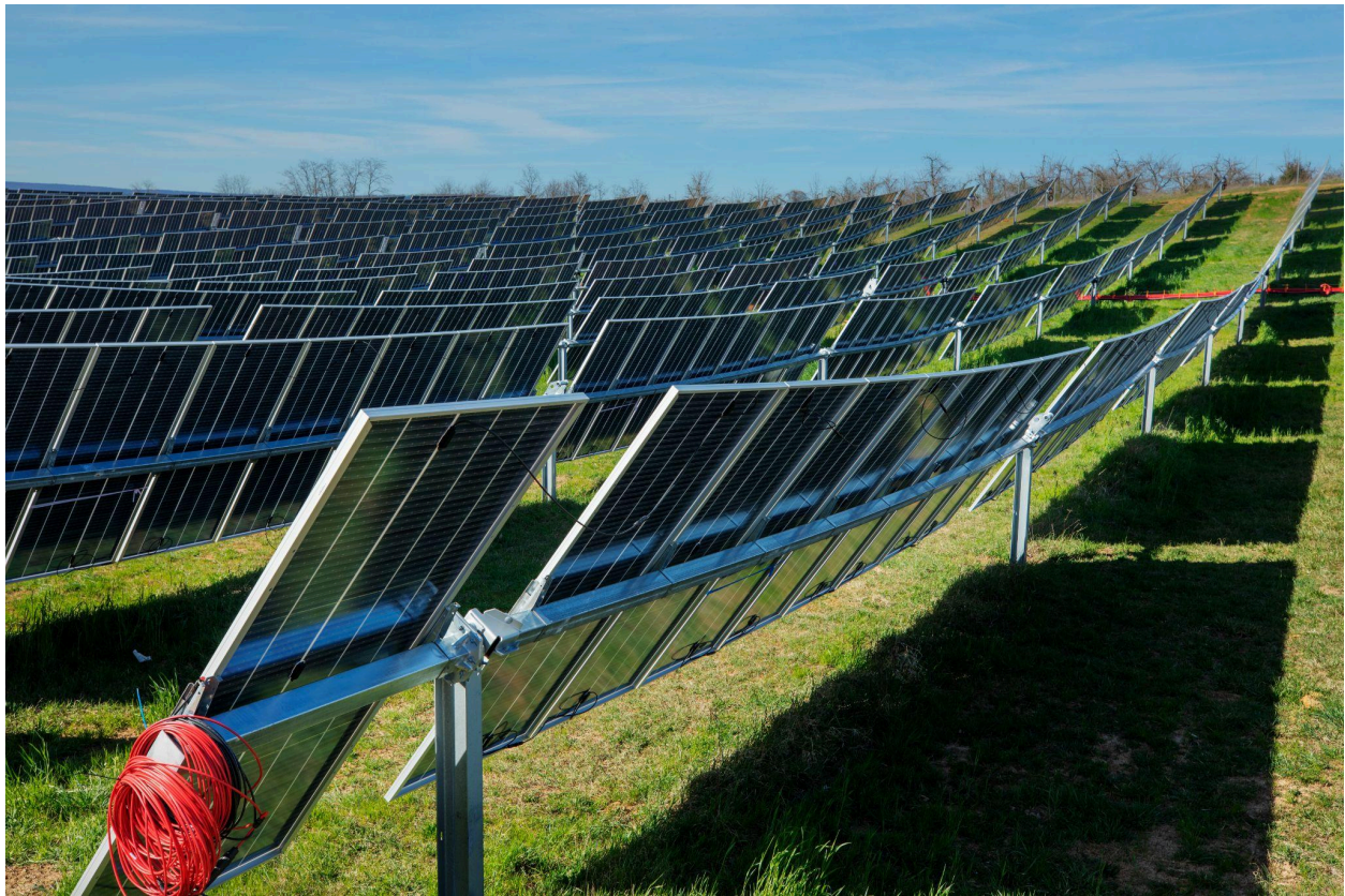
Nevados All Terrain Trackers, precommissioning at the Bartonsville Energy Facility in Virginia. Photo: Nevados
