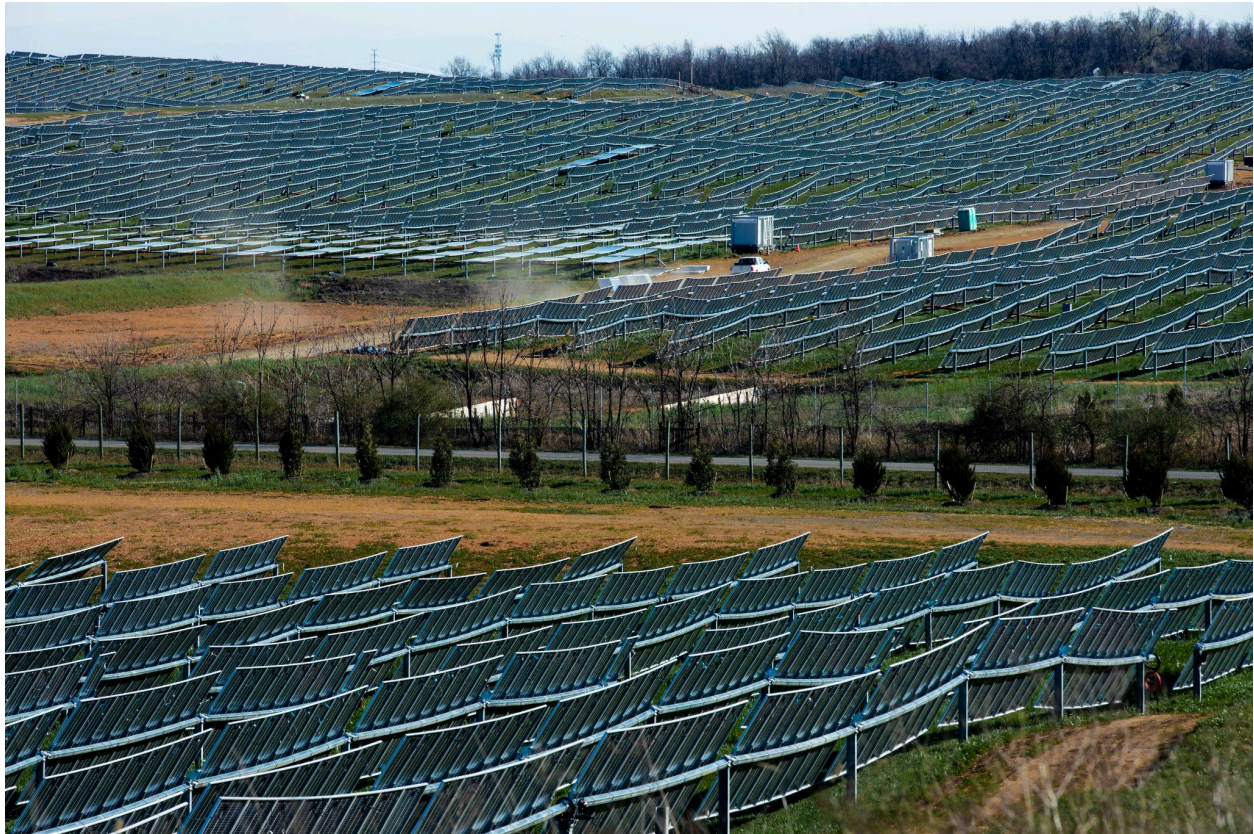
Nevados All Terrain Trackers awaiting commissioning at the Bartonsville Energy Facility, a 170 MW solar farm near Winchester, Virginia. Photo: Nevados
